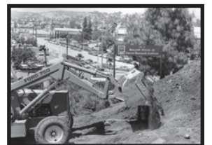
Heavy construction equipment clears ground for the USC Norris Comprehensive Cancer Center.
